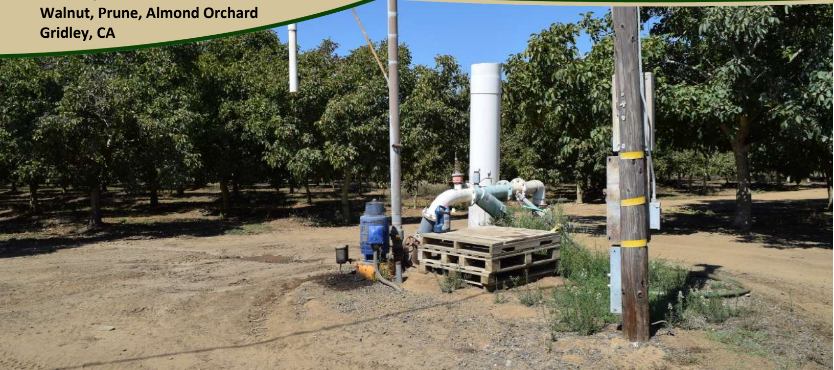
30 HP Irrigation Well
