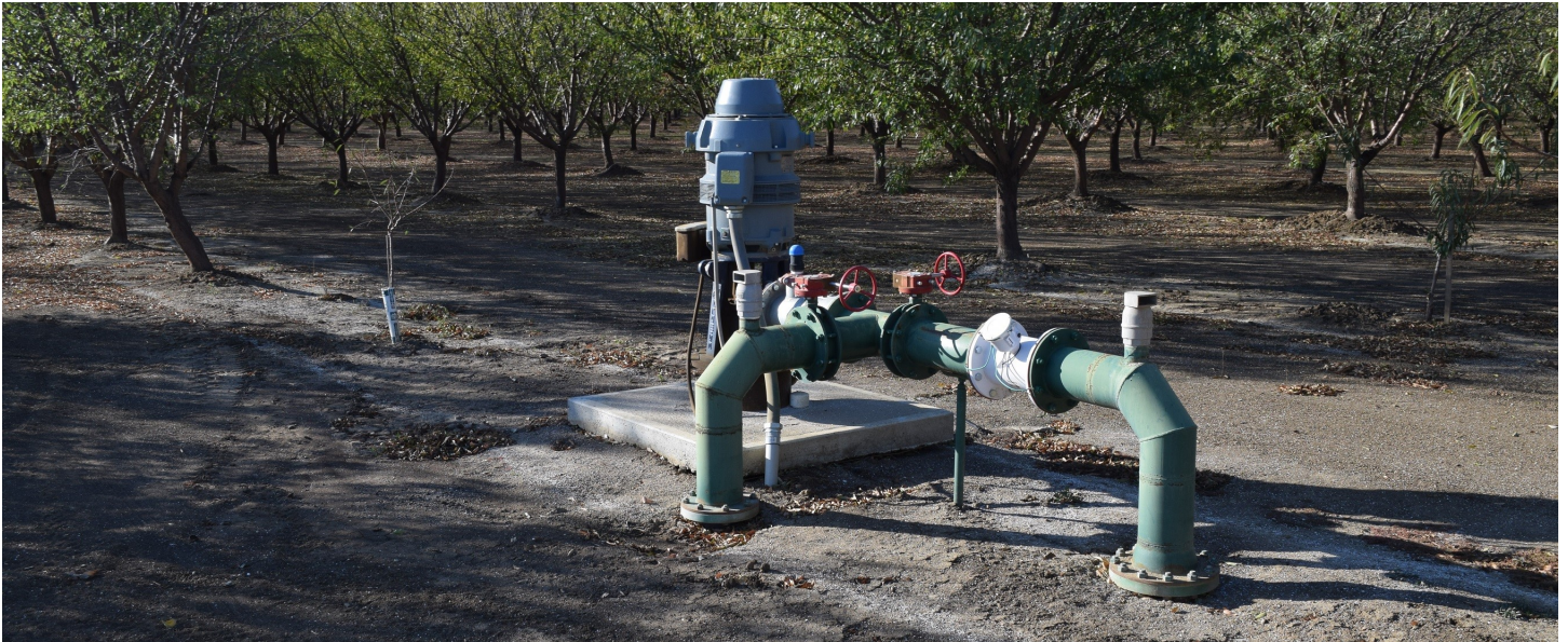
Lift pump, filter station with well tie in
