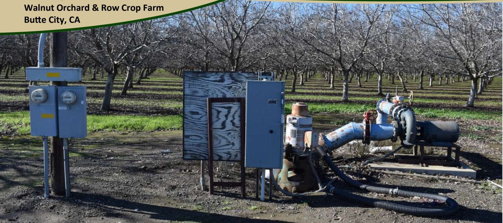
Irrigation Well & Booster Pump in Block #1
