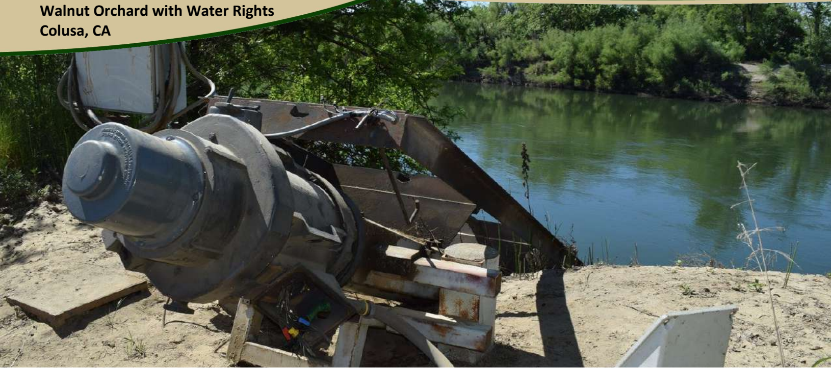
River Pump and Fish Screen
